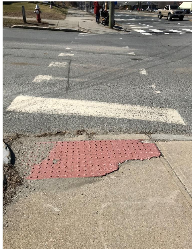
Deteriorating Street Crossing Source: Hodge Economic Consulting
