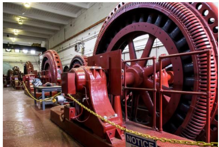
Turners Falls Hydroelectric Station Photo: FirstLight Power
